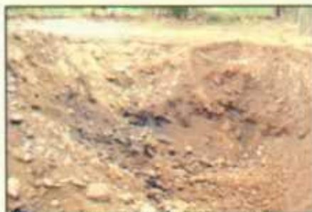
Hydrocarbon stained soil on west wall
