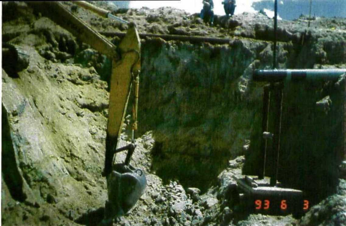
REMAINING SOIL CONTAMINATION- SOUTH WALL-BENEATH 8" PIPELINE
