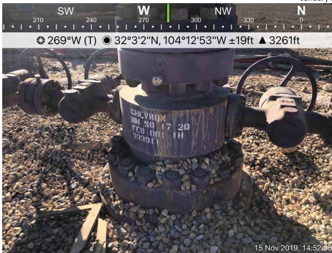
Chevron HH SO 17 20 Federal 001, November 15, 2019
