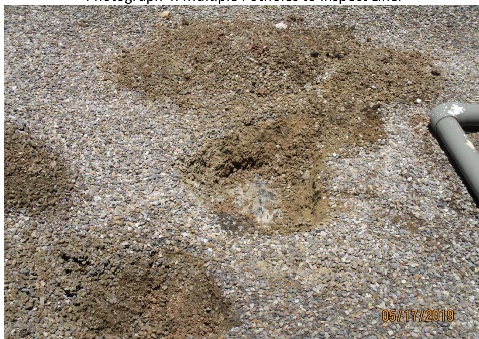
Photograph 4: Multiple Potholes to Inspect Liner
