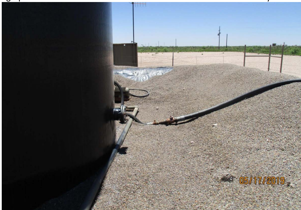
Photograph 2: Lea KG State New Produced Water Tank and Clean Secondary Containment
