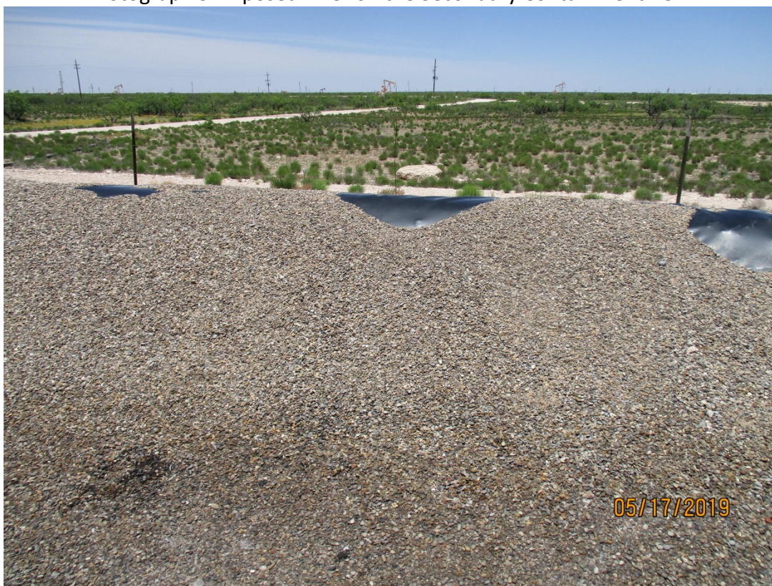
Photograph 5: Exposed Liner on the Secondary Containment Berm
