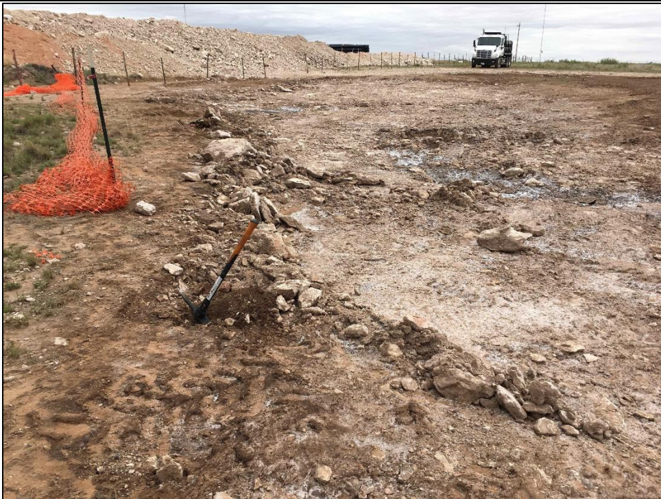
PHOTO 28: View of CS-17, Facing Southwest. 6/10/2019 / TIME: 2:19PM / GPS: 32.5254 -103.5207
