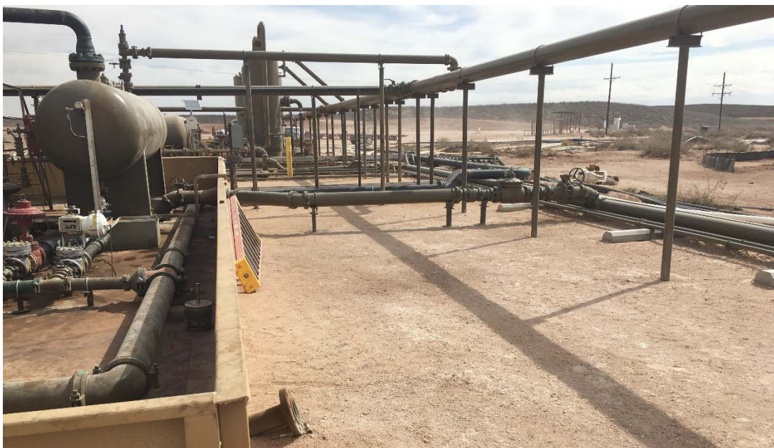
Photograph 1: View of process equipment area.
