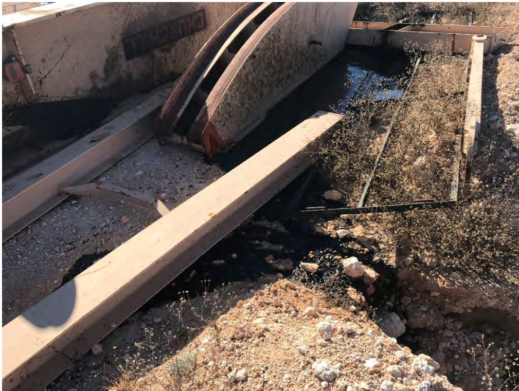
Release (Looking West-Southwest)
