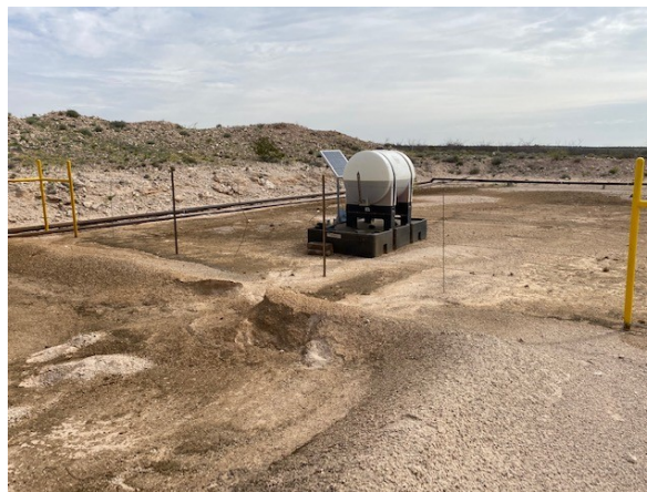
Photograph 2: View of breached earthen berm and staining in northeast corner of well pad.
