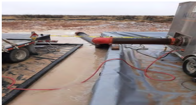
Photo 1: View southwest of disconnected lay flat line
