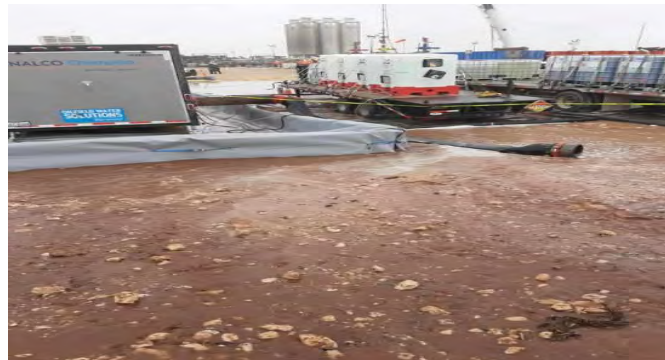
Photo 2: View northwest of disconnected lay flat line and equipment
