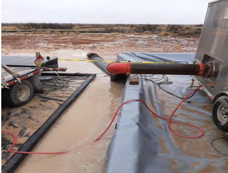
Photograph 1: Southwest view of disconnected lay flat line.
