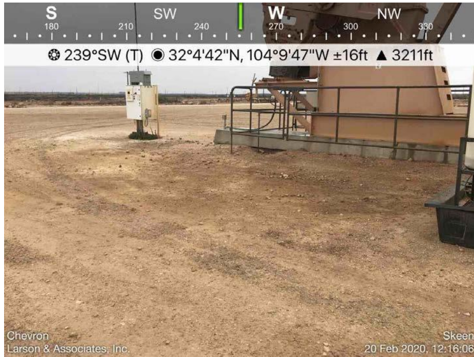
Impacted area viewing west/southwest, February 20, 2020
