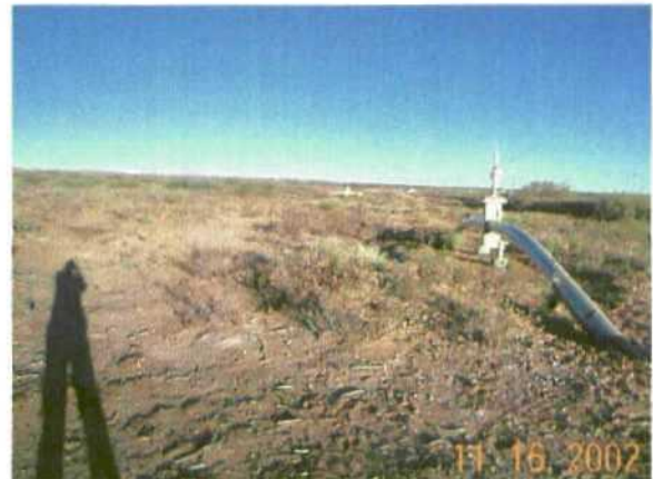
Photo 5. Pipeline ride-of-way west of the landfarm facility. Contaminated soil found in the pipeline ride-of-way.
