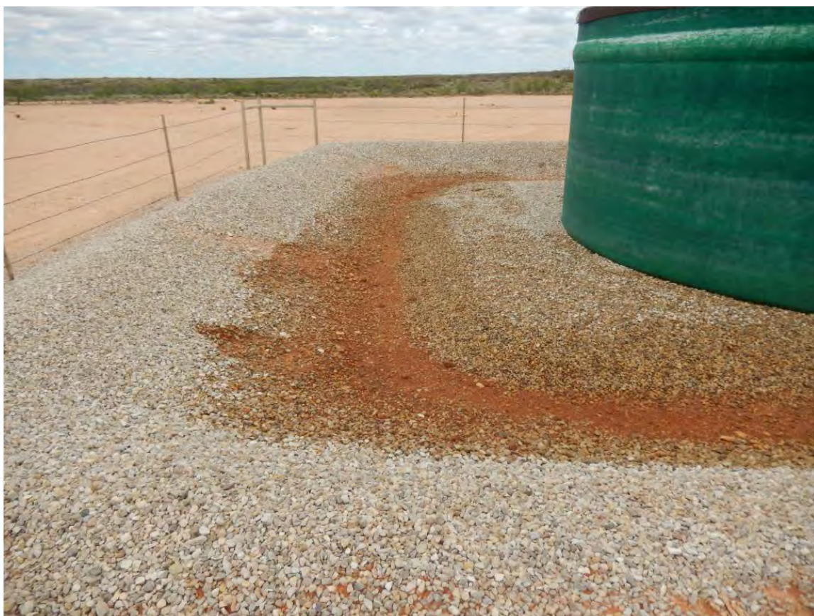
Stained Area inside firewall facing North, June 1, 2016
