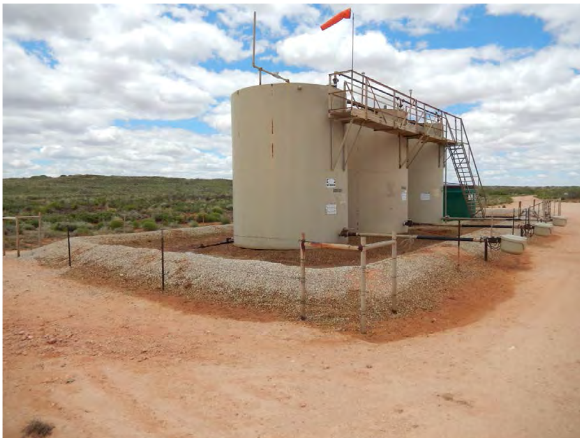
Stained Area inside and outside firewall facing Southeast, June 1, 2016
