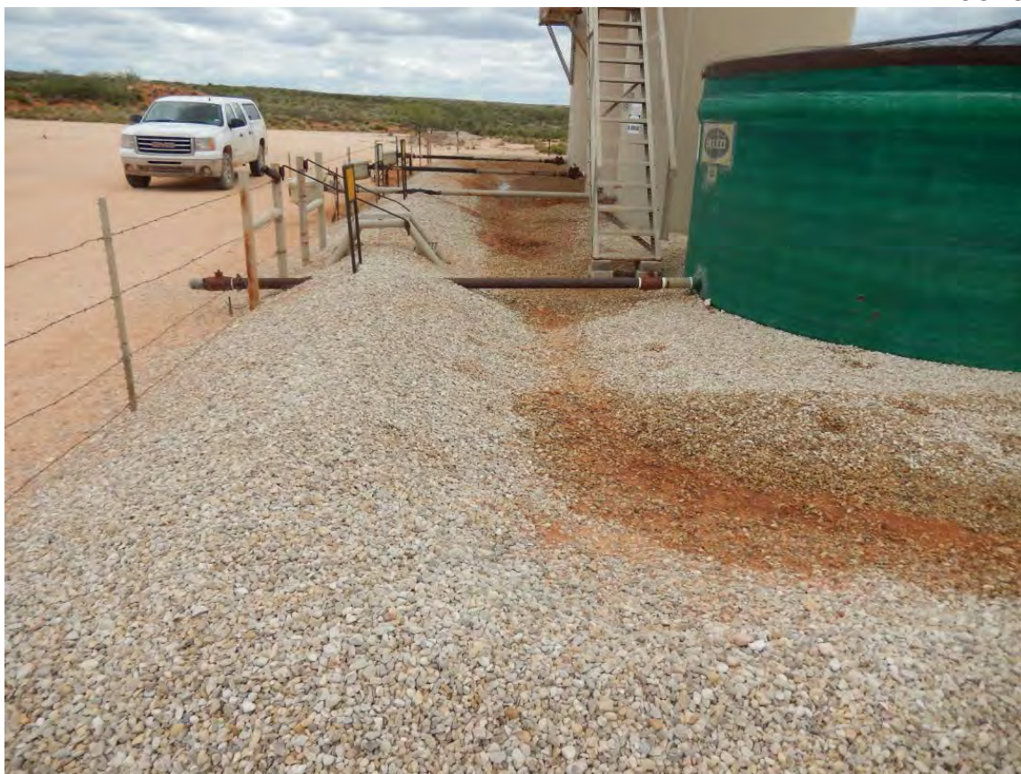
Stained Area inside firewall facing East, June 1, 2016
