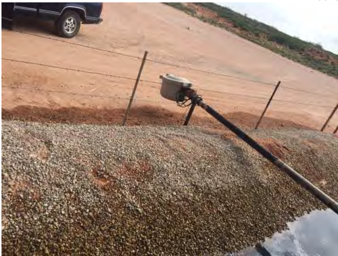
Stained Area outside firewall North of Tanks facing Northeast, May 30, 2016
