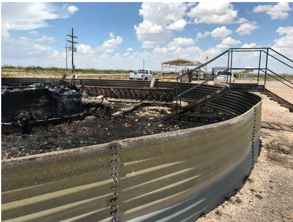
Indian Basin Station 210 – Release (Looking North)
