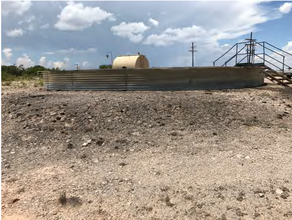
Indian Basin Station 210 - Release (Looking West)
