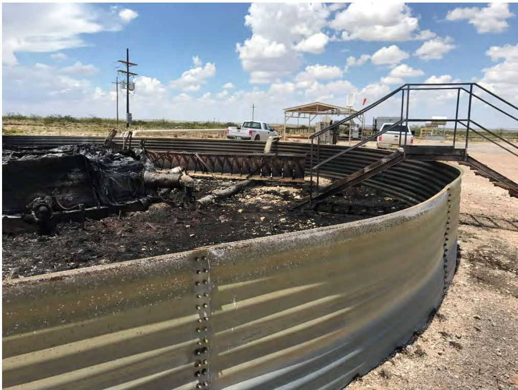
Indian Basin Station 210 – Release (Looking North)
