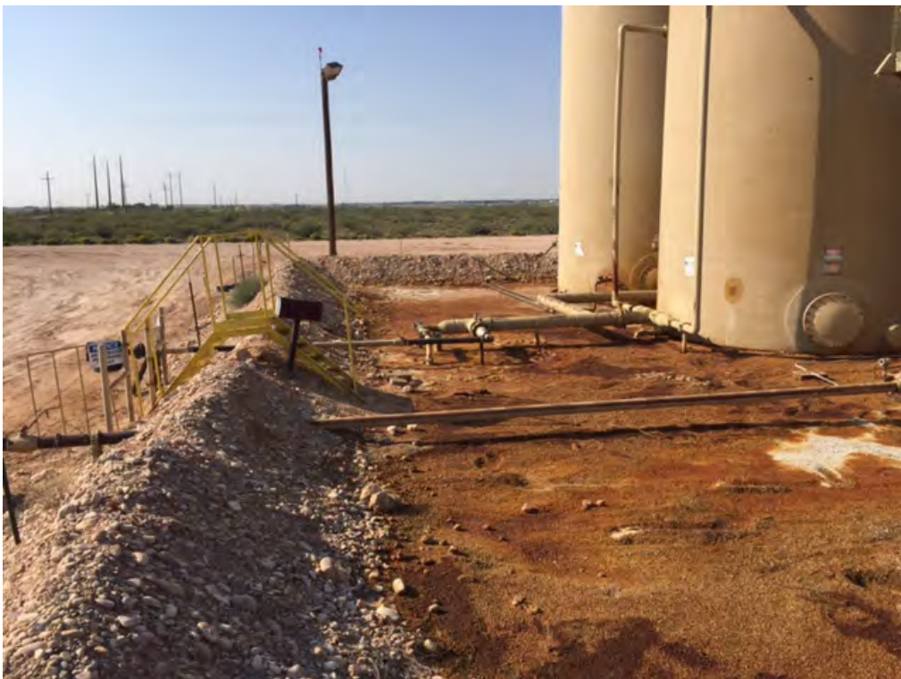
NEL 4 SWD Battery - Release (Looking South)
