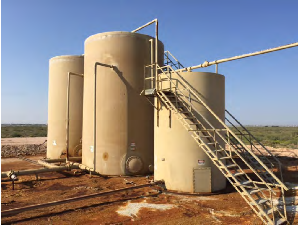
NEL 4 SWD Battery - Release (Looking South-Southwest)
