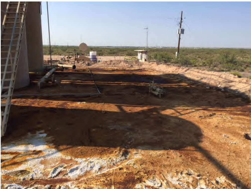
NEL 4 SWD Battery – Release (Looking South)
