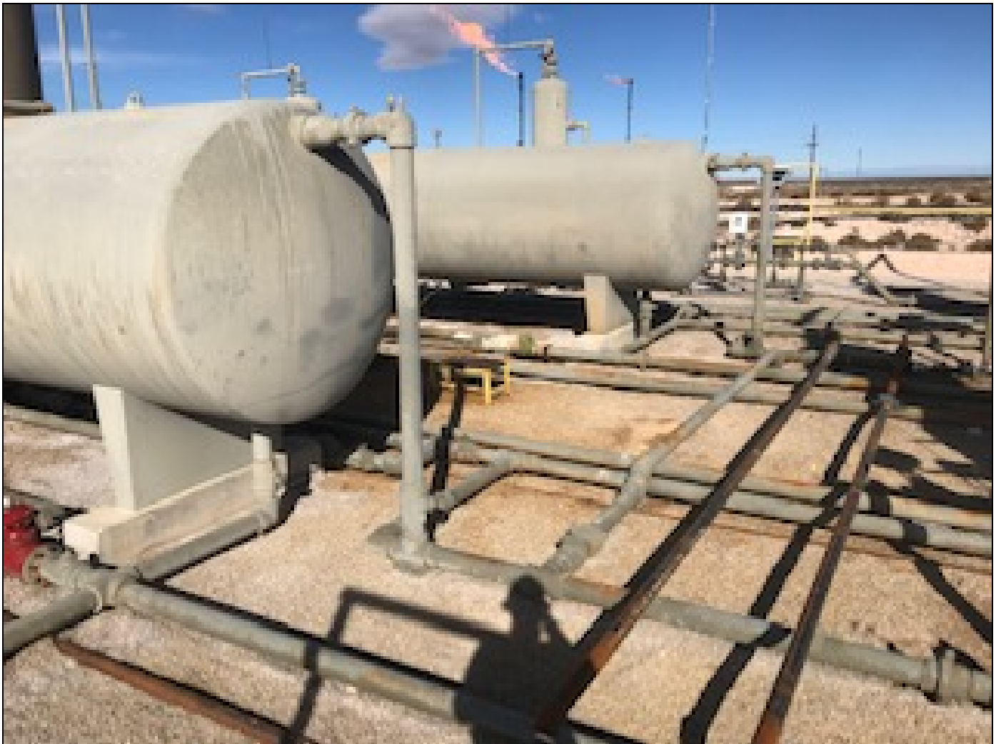
View northeast of free-water knockout tanks and soil impacts around piping.
