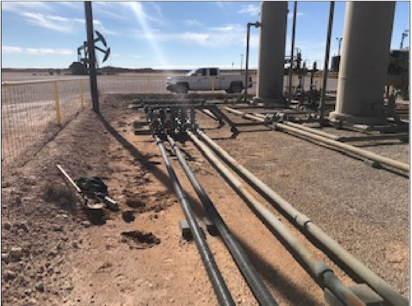
View south showing piping density in release area.
