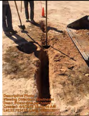
Power-line pot holed
