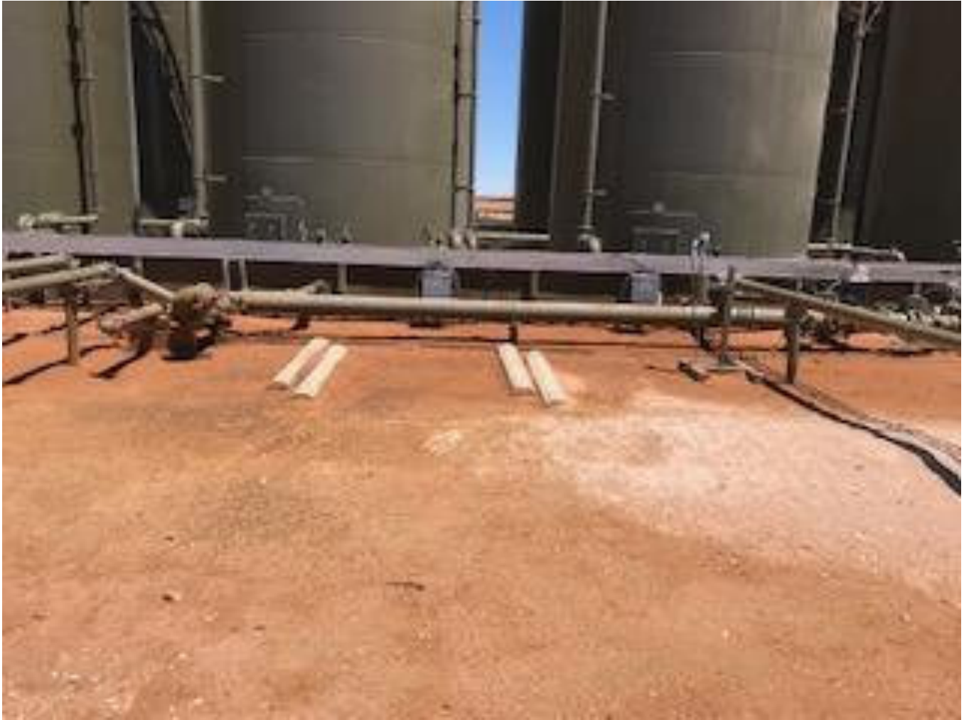
Northern view of point of release area and tank battery containment during site assessment activities.
