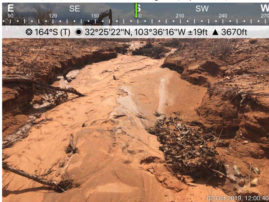
Water Eroded Channel Viewing South, October 2, 2019
