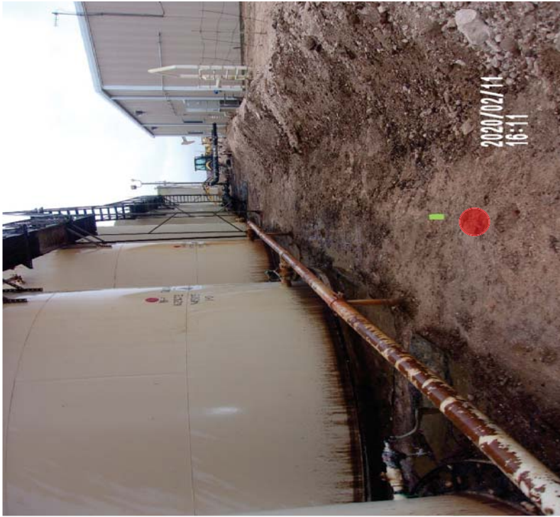
View West - Sample location Auger Hole 3 (1' EB) (red circle) middle of photograph.
