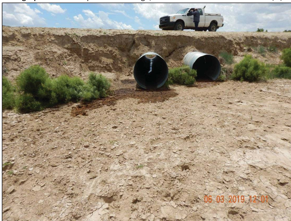
Photograph 6: Visual Impacts to Drainage; Down-Gradient from Culverts – 6/3/19
