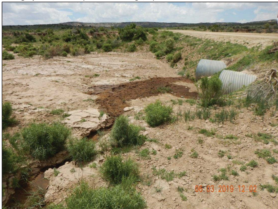
Photograph 5: Visual Impacts to Drainage; Up-Gradient from Culverts – 6/3/19
