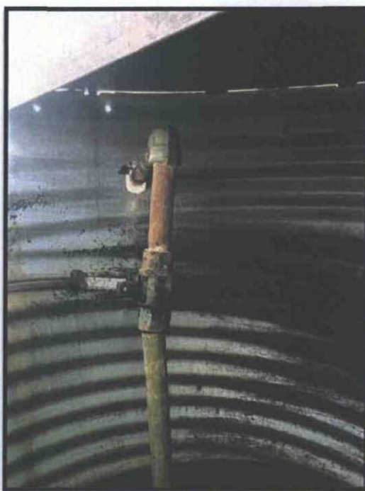
Photo of the NEBU 454A valve in the valve can that is the source of the spill.
