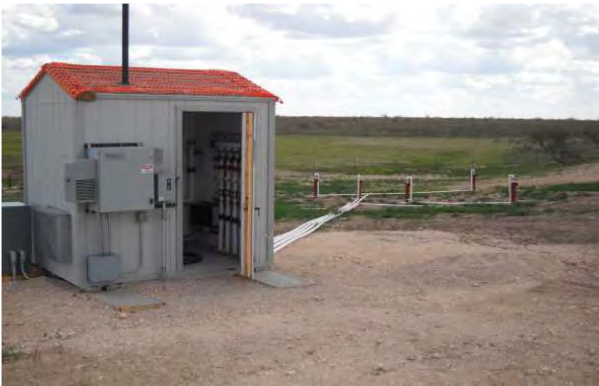
EK Queen Pearce 6-Inch – SVE System Housing & Extraction Wells
