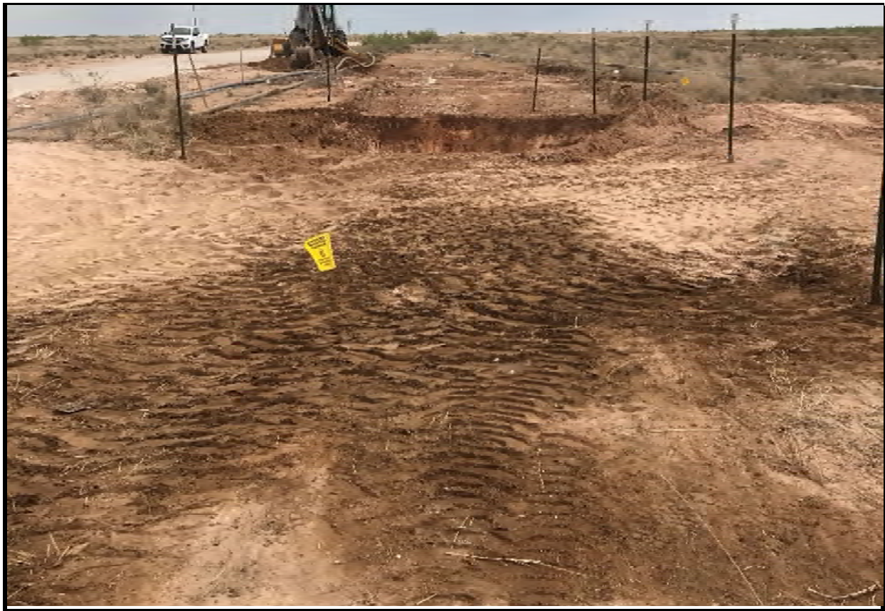
Figure 1 - View of affected area and partial excavation, facing Northeast.
