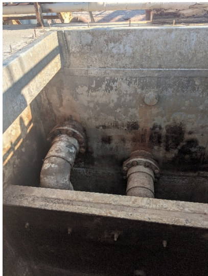
Photo 3. API – East Bay, North End, Hole Located Above Left Pipe
