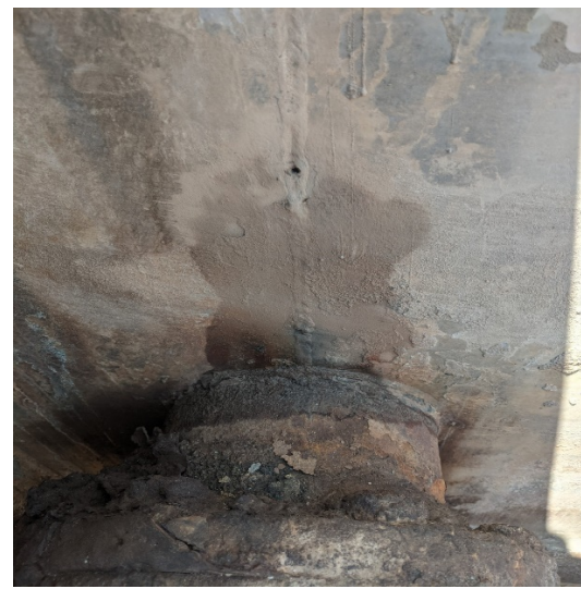
Photo 4. API – East Bay, North End, Hole Above Pipe
