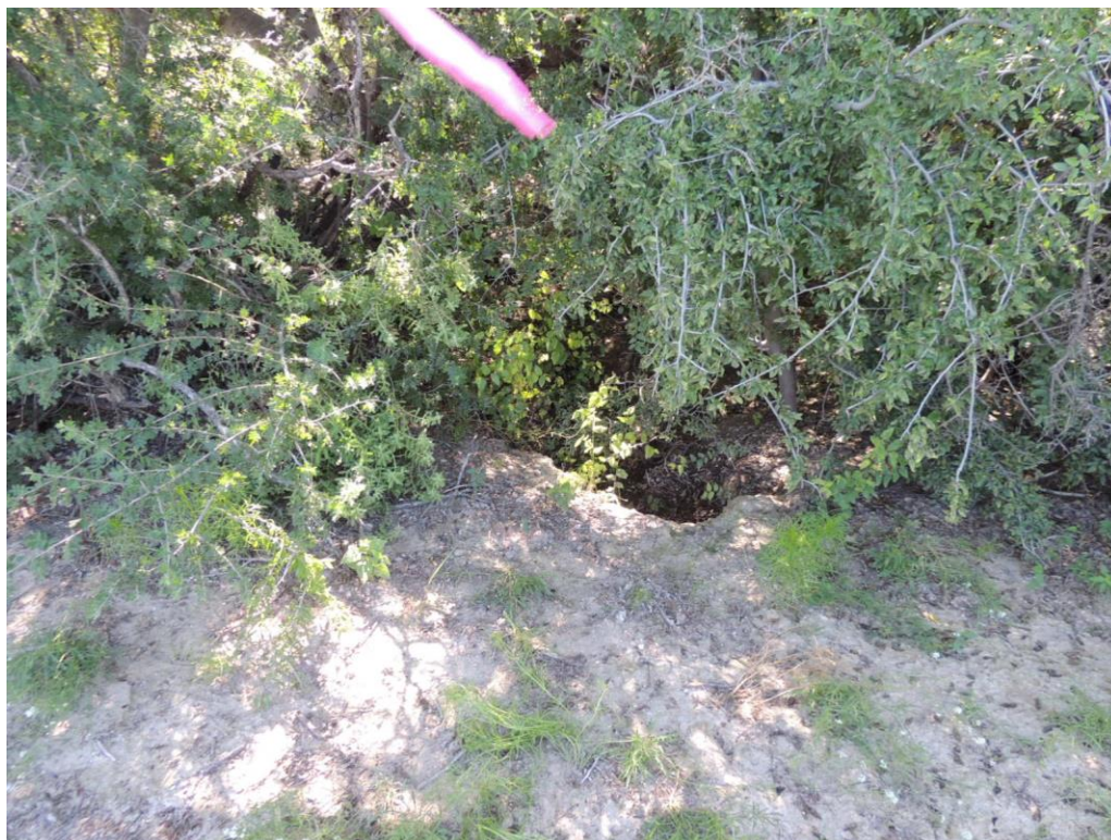
SURFACE DEPRESSION WITH DRAINAGE HOLE 564669E, 3543067N
