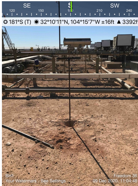
View of Pump Area— View South
