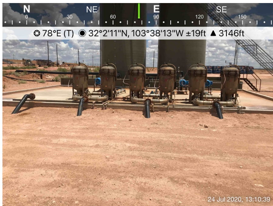
View of the equipment to the west of the spill area.
