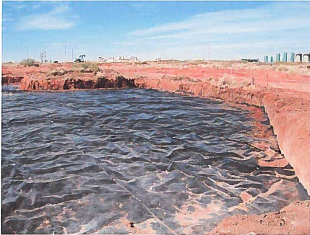
View West – Along COG buried water line at SB-1 and SB- 5
