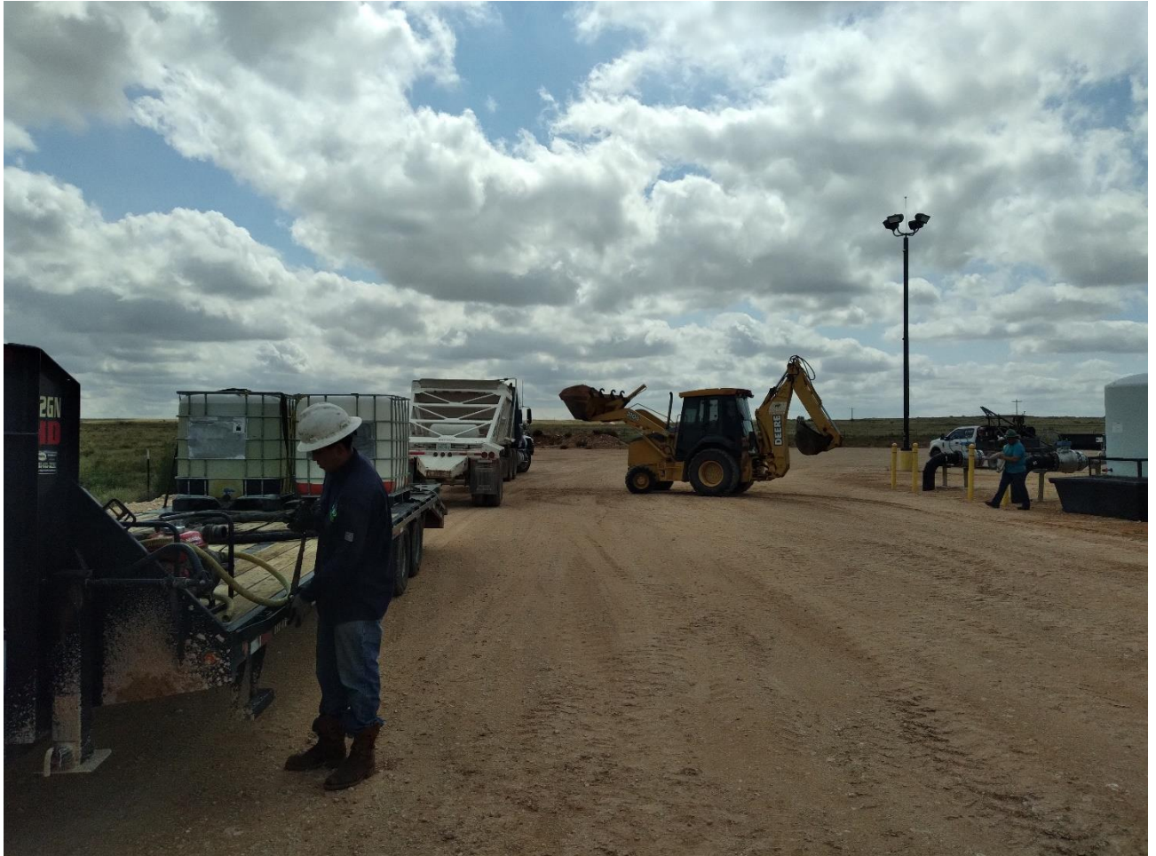
Figure 7: Removal of Top Layer of Contaminated Soil Using Backhoe and belly-dump trucks
