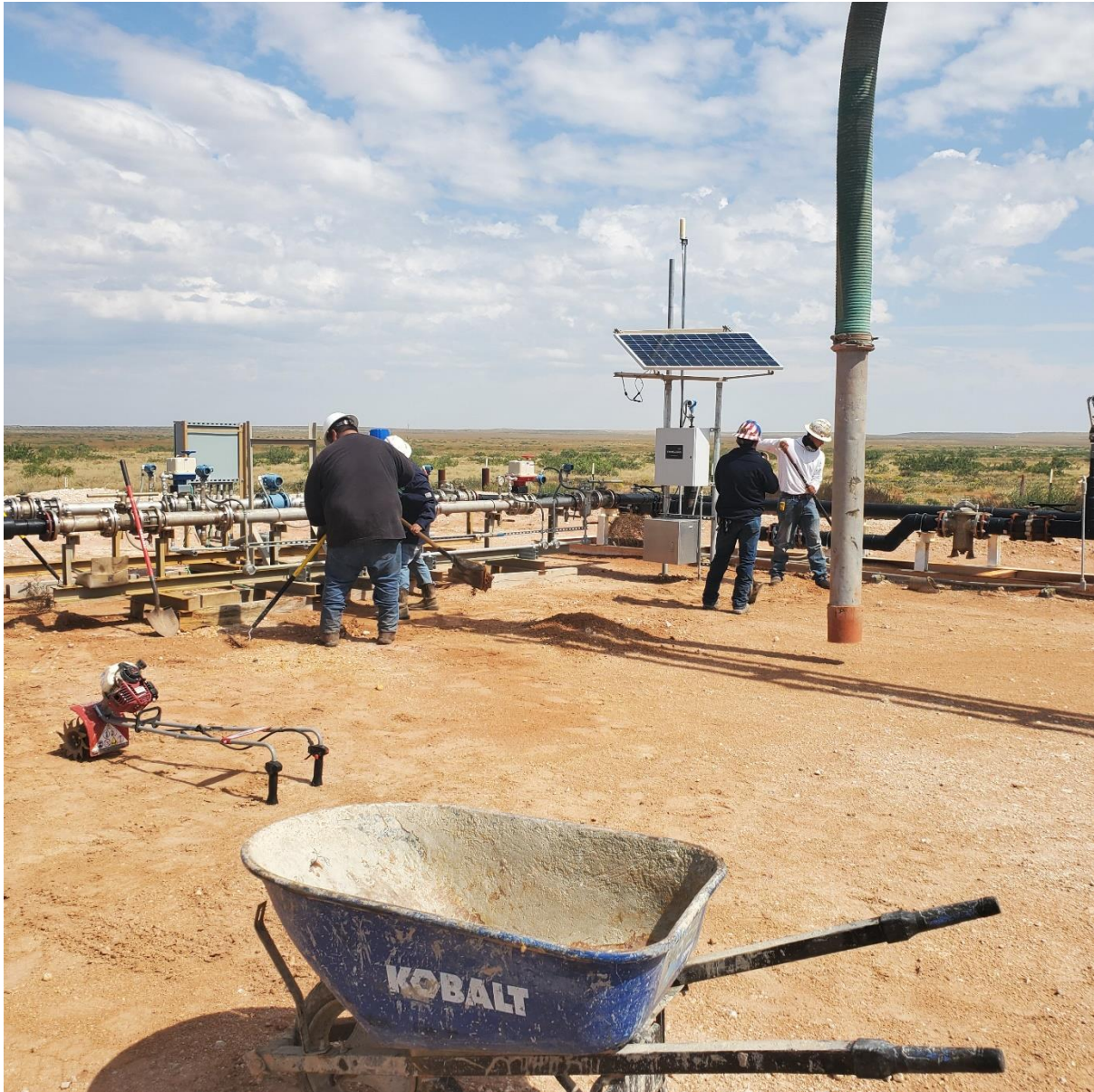
Figure 4: Removal of Top Layer of Contaminated Soil Near Pipes of Location Cheddar RP SWD
