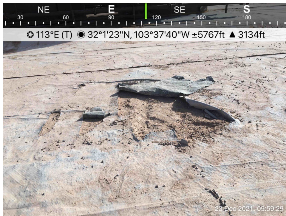
View of torn liner, December 23, 2021
