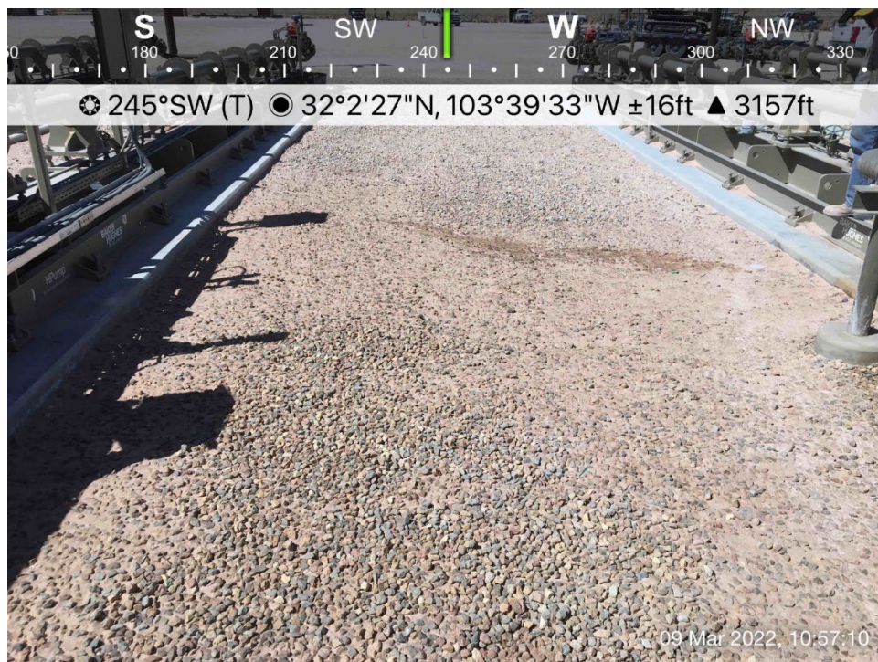
Impacted area viewing southwest, March 9, 2022
