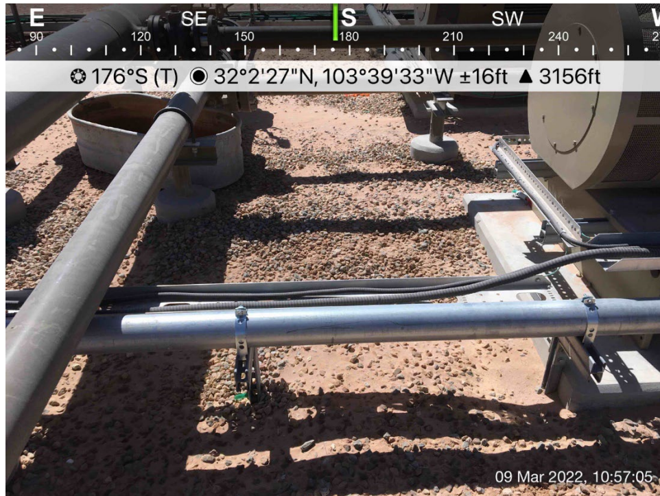
Impacted area viewing south, March 9, 2022
