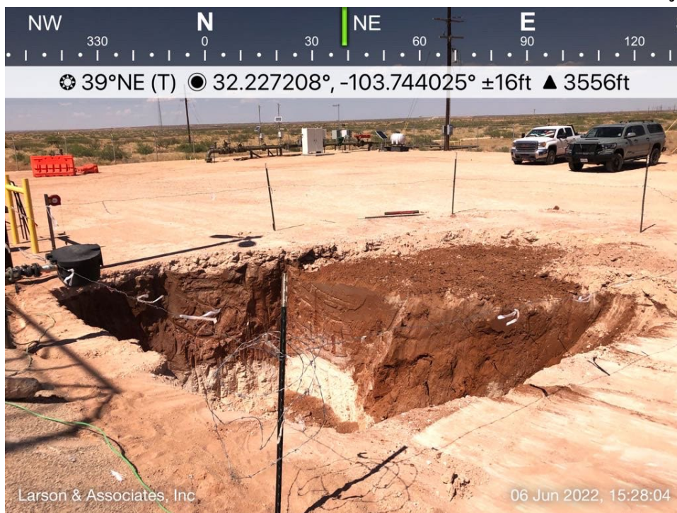
Excavated soil (nAPP2106659781) viewing Northeast
