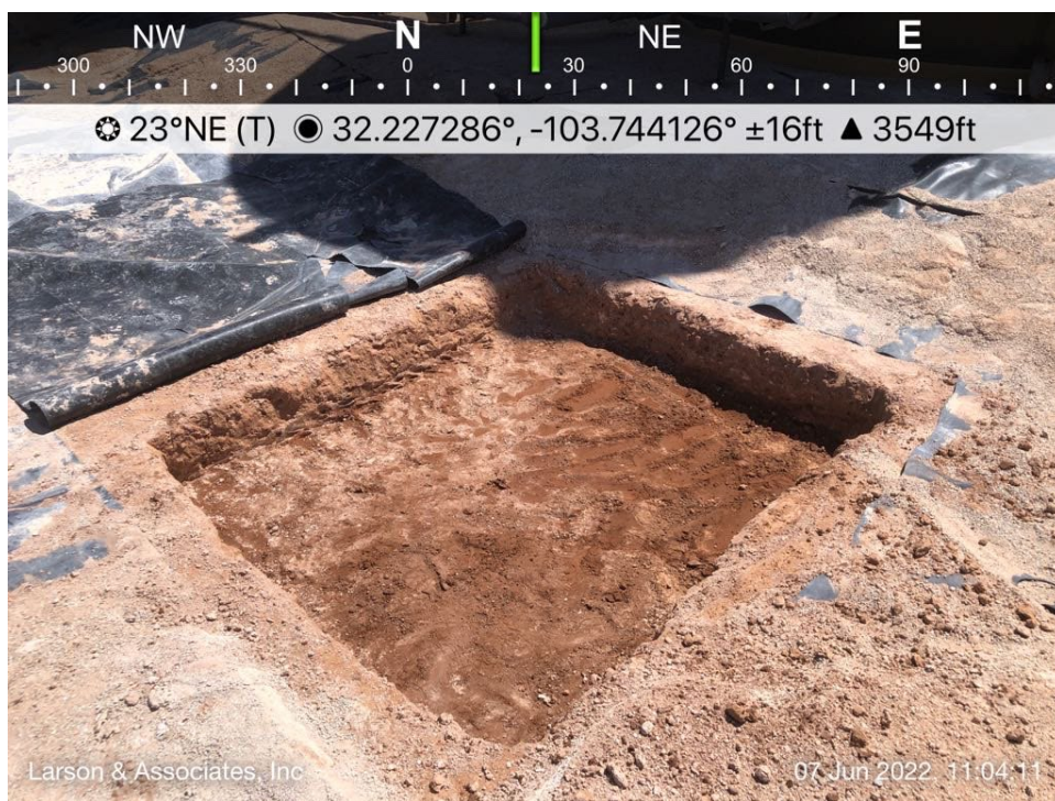
Excavated soil (nAPP2205652777) viewing Northeast
