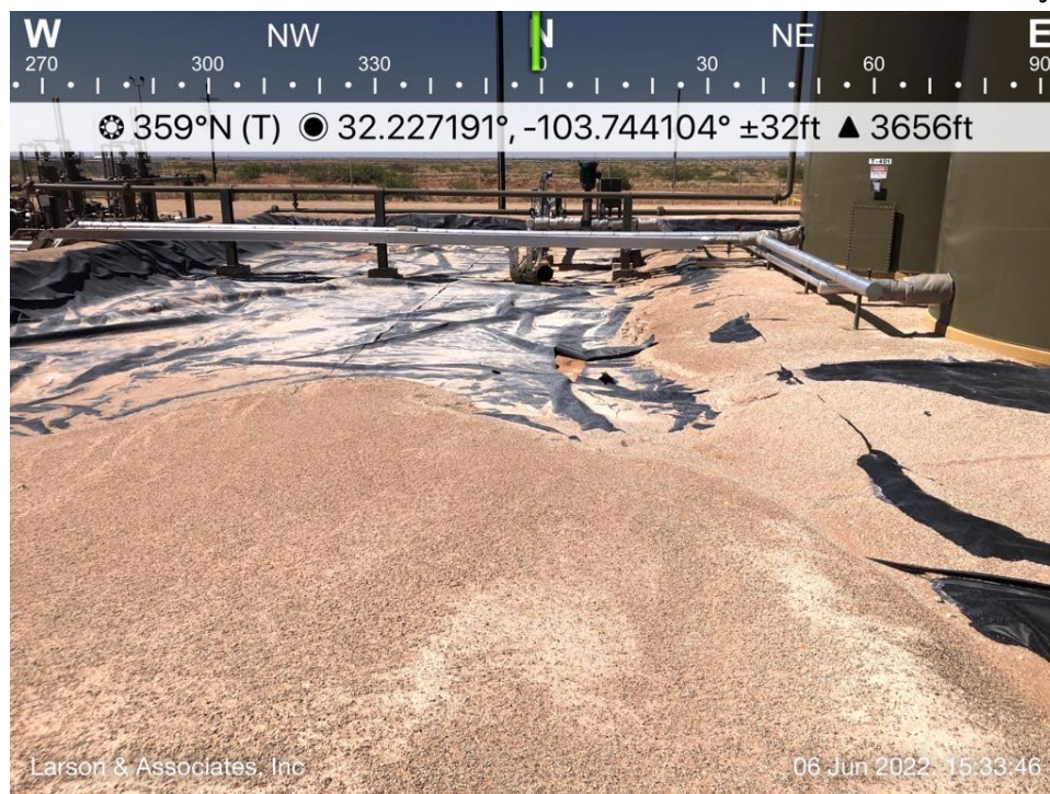
Torn Liner (nAPP2205652777) viewing North
