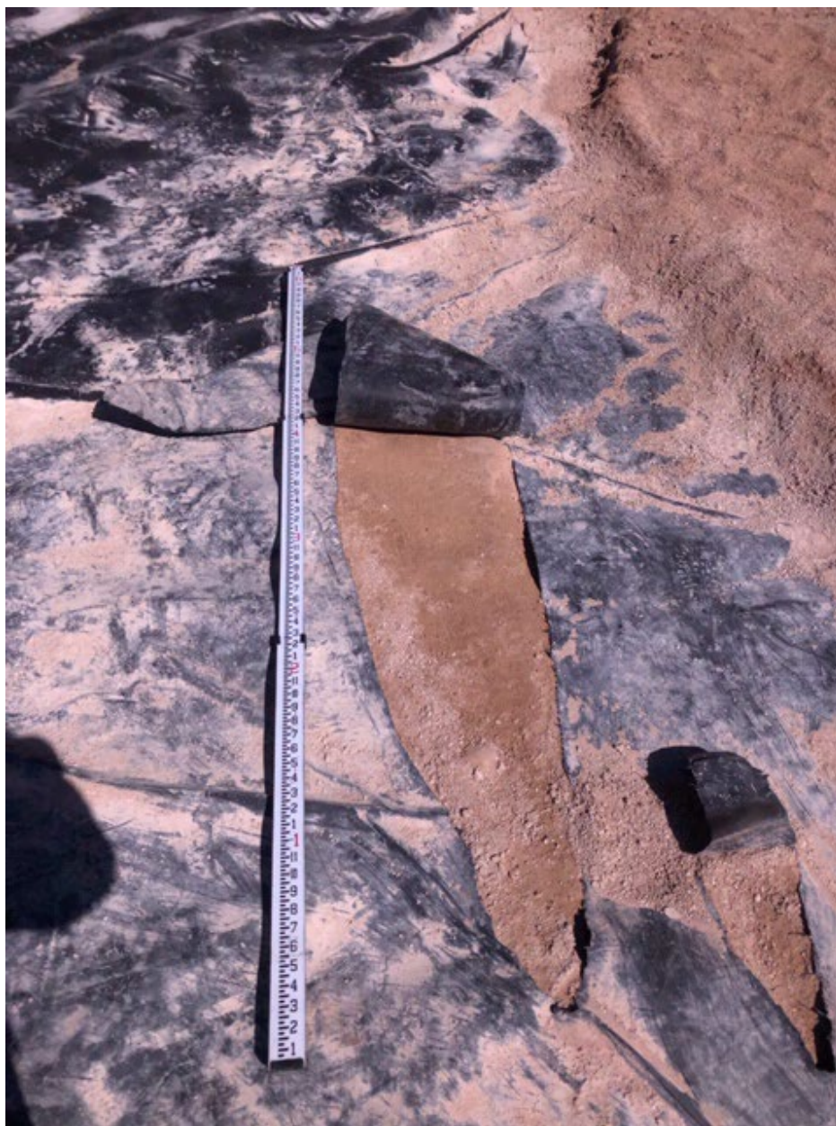
Torn liner (nAPP2205652777) viewing North
