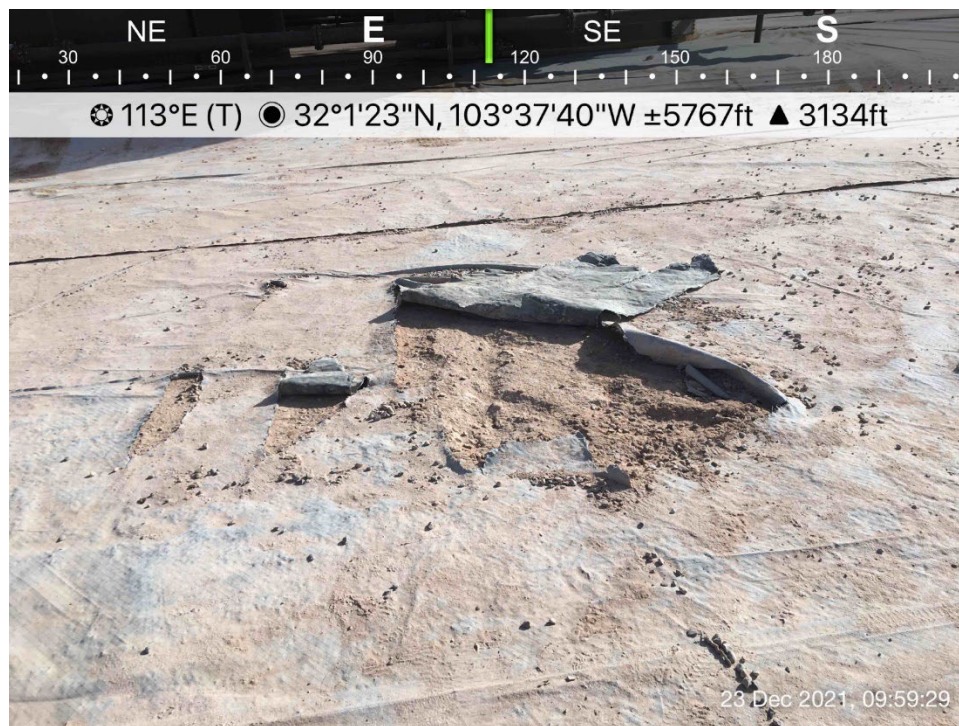
View of torn liner, December 23, 2021
