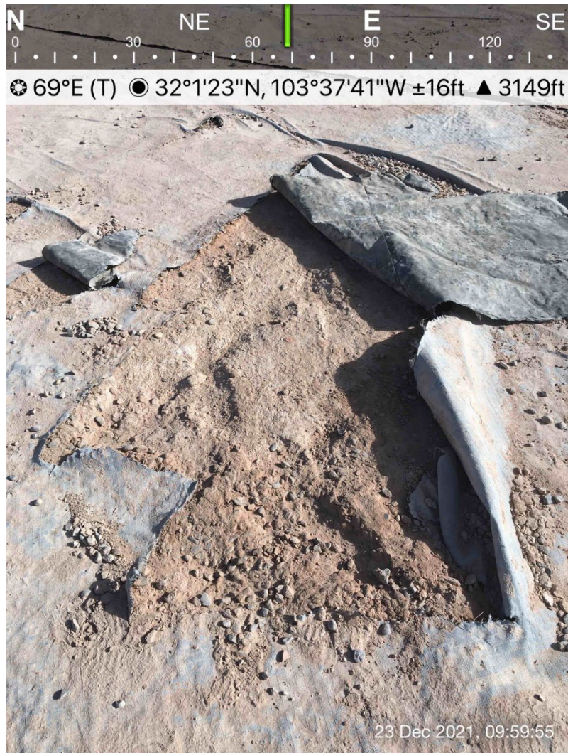
View of torn liner, December 23, 2021
