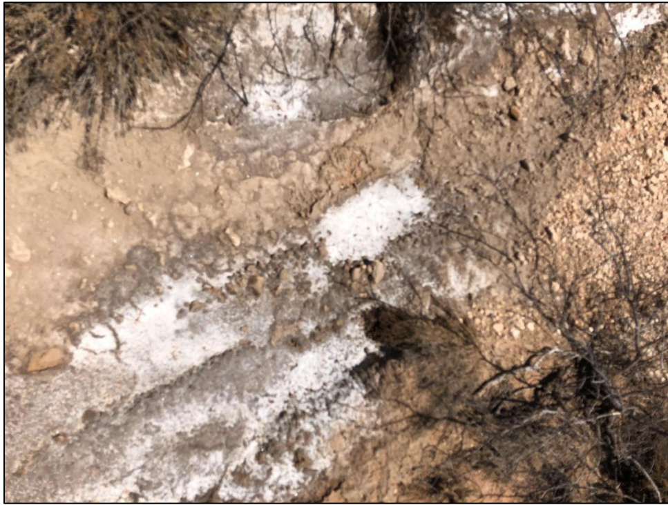
PHOTO 13: View of staining and width of flow path. 7/15/2019
