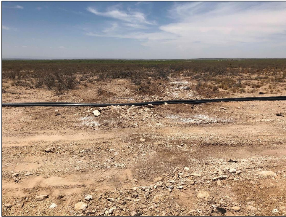
PHOTO 11: View of sight and staining going into drainage, facing west. 7/15/2019
