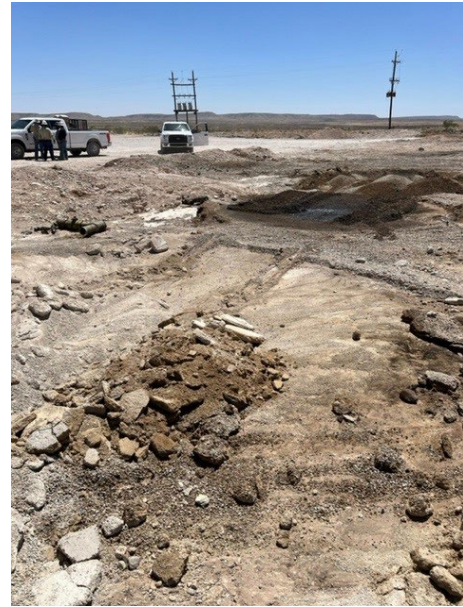
Photograph 2 Date: 18-May-22 Description: View of staining observed following tank removal facing south.
