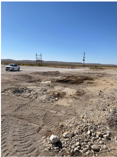
Photograph 3 Date: 28-Apr-22 Description: View of containment showing all tanks removed, facing south.
