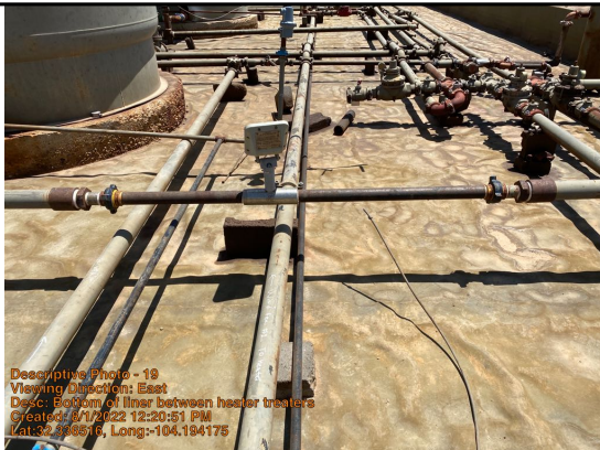
Bottom of liner between heater treaters
