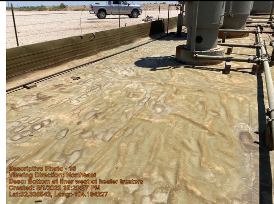
Bottom of liner west of heater treaters
