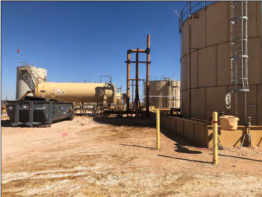
PHOTO 2: View of the impacted area facing north. 9/29/22
