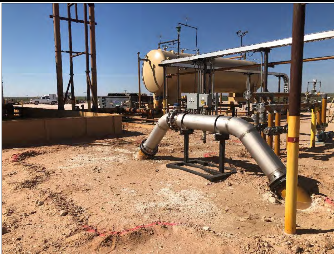
PHOTO 4: View of the impacted area facing southwest. 9/29/22
