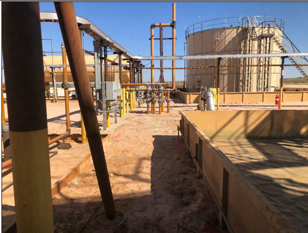
PHOTO 3: View of the impacted area facing north. 9/29/22
