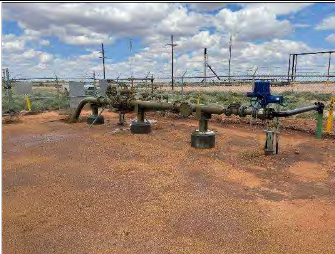
PHOTO 3: View of the impacted area facing northeast. 8/25/22
