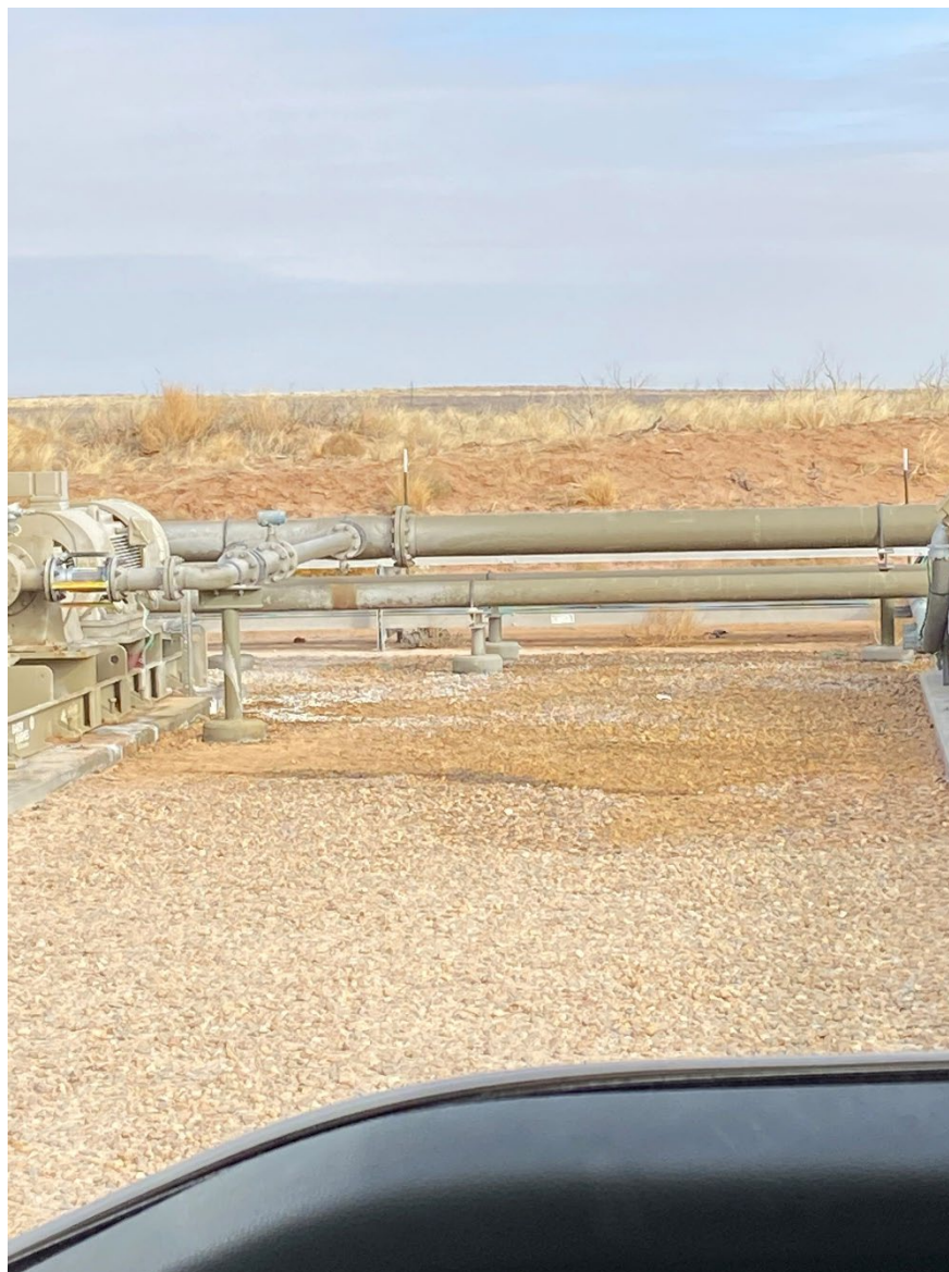
Impacted area (nAPP2202549943) captured by Chevron personnel
