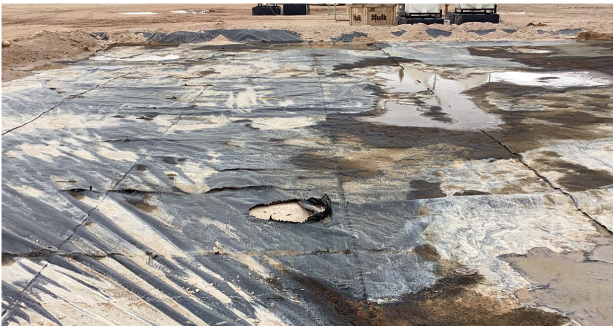
Photo 8 View of a damaged and impacted lined area within the Earthstone pad, which is not related to the Delek Release..
