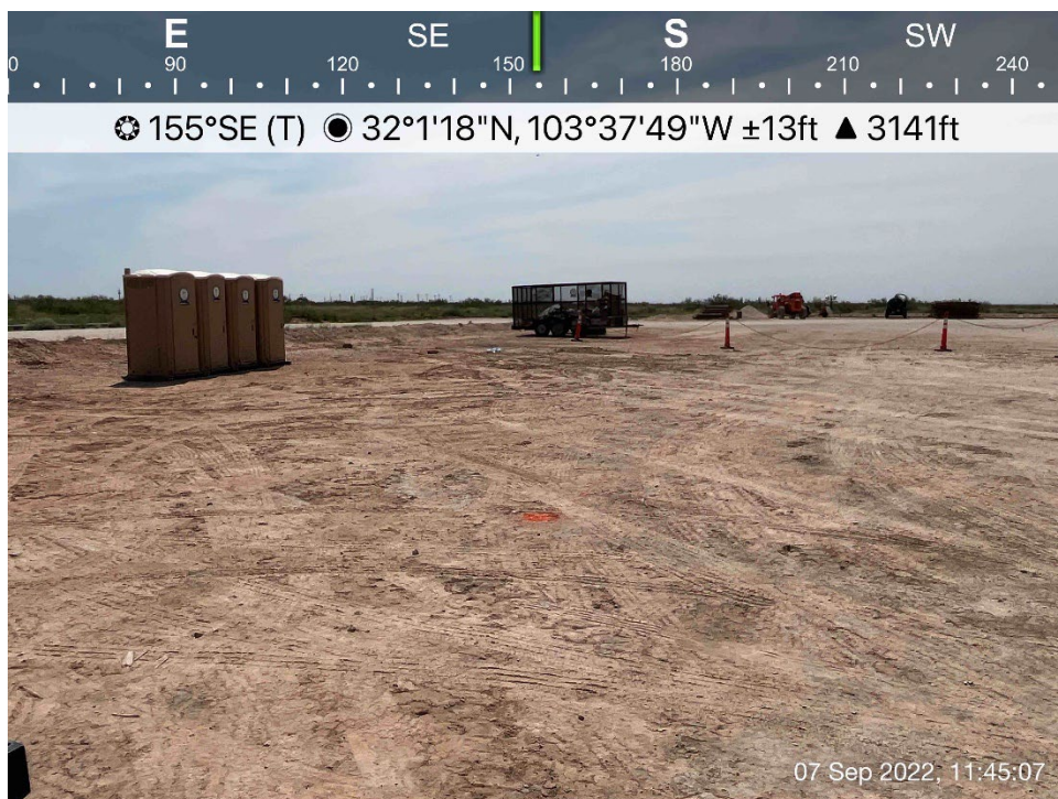
Impacted area viewing south/southeast, September 7, 2022
