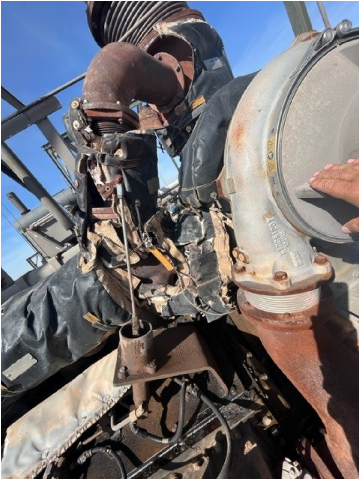
Photo 2: View of equipment that caught fire.
