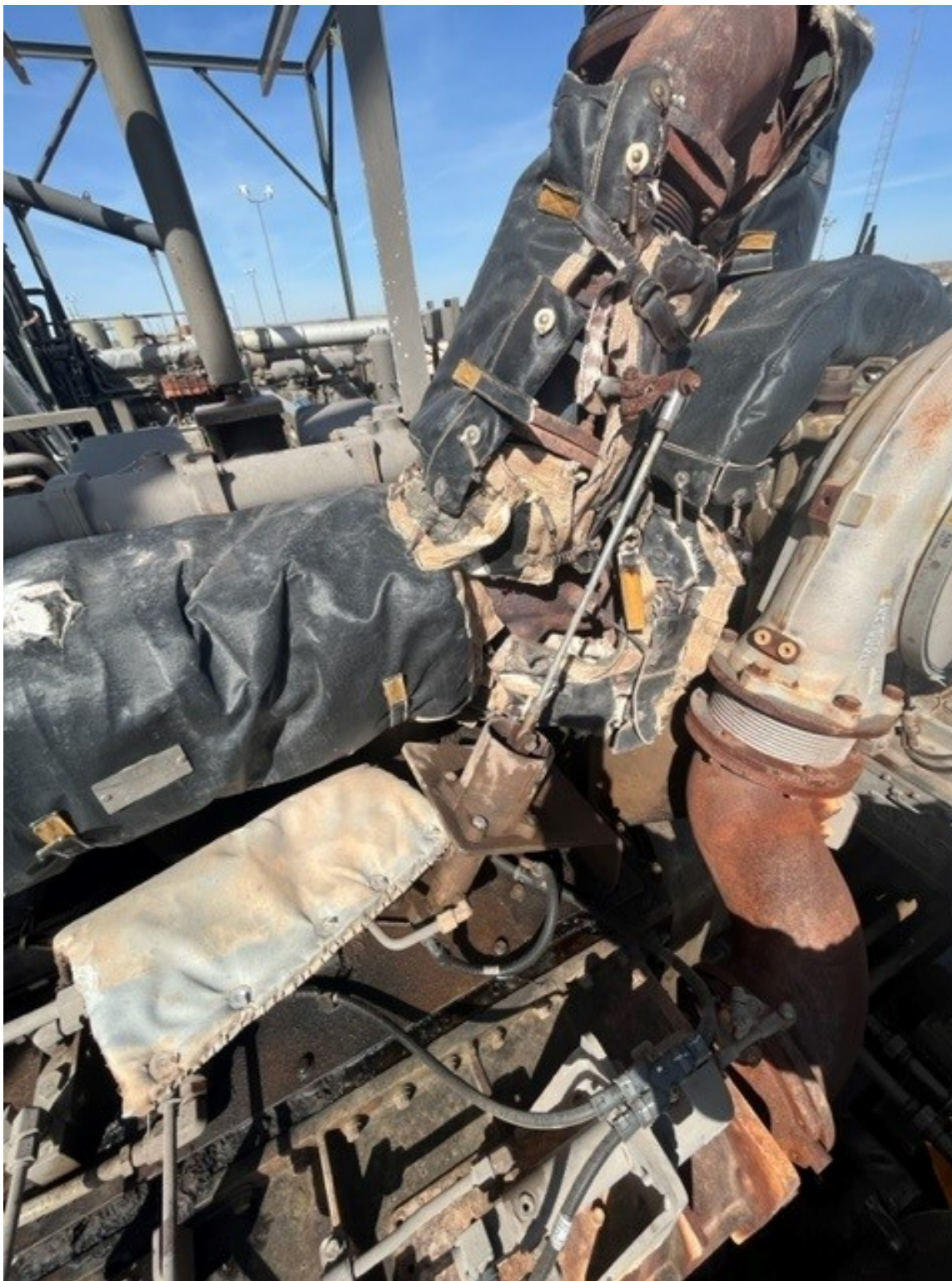
Photo 1: View of equipment that caught fire.
