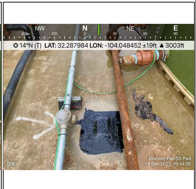
Photograph 4 Description: Patched Liner View: North
