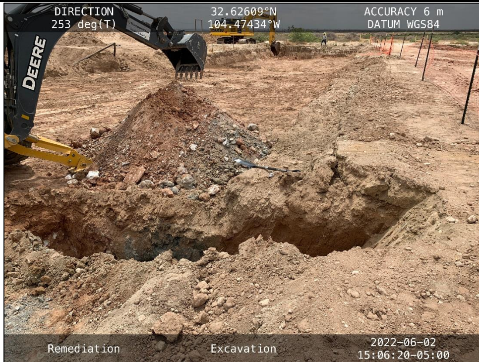
PHOTO 32: View of remediation around the tank battery, facing west.
