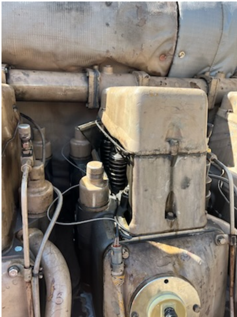
Photo 2: View of equipment that caught fire.
