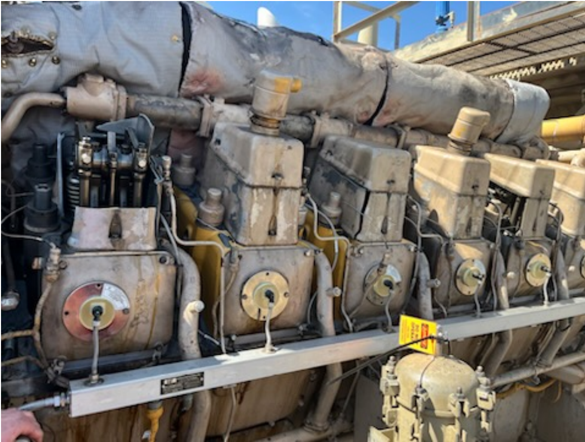
Photo 1: View of equipment that caught fire.
