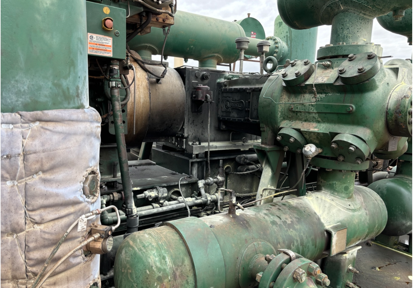
Photo of Property Damage to the Compressor
