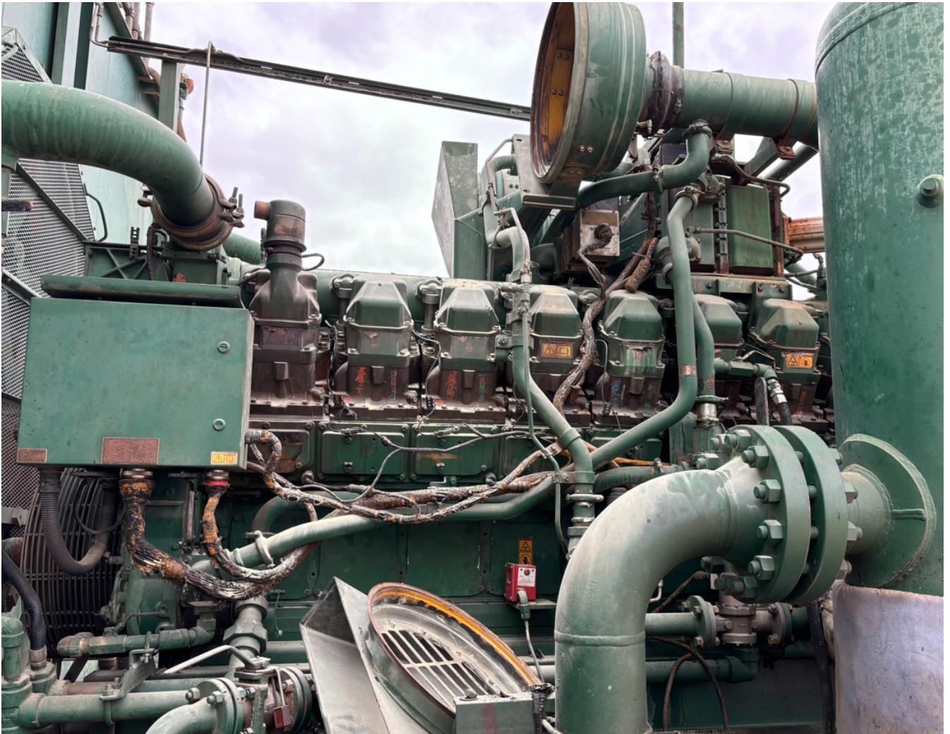
Photo of Property Damage to the Unit Wiring and Insulation
