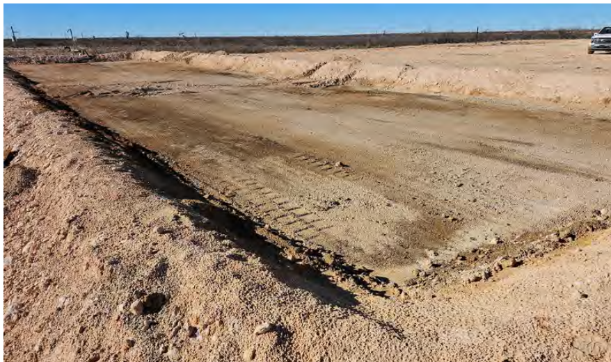
Figure 1: View of tank battery footprint following deconstruction facing northwest from the southeast extent. Date Taken: 2023-12-27 13:52:05. GPS: 32.388770, -103.190065
