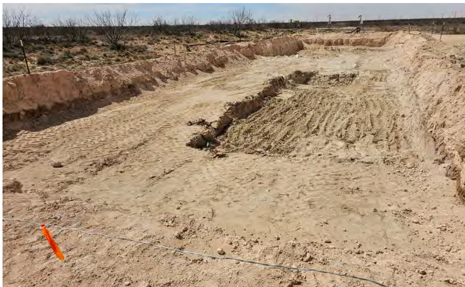
Figure 2: View of final excavation extent facing southwest from the northeast extent. Date Taken: 2024-03-06 12:10:40. GPS: 32.388791, -103.190034.
