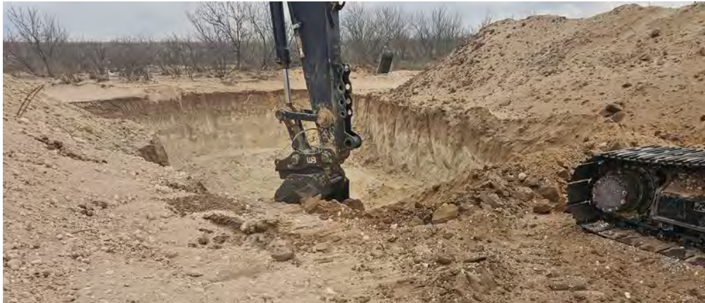
Figure 4: View of excavation trench being expanded to encapsulate trench per SLO approved Reclamation Plan. Date Taken: 2024-03-25 14:11:21. GPS: 32.388987, -103.190264
