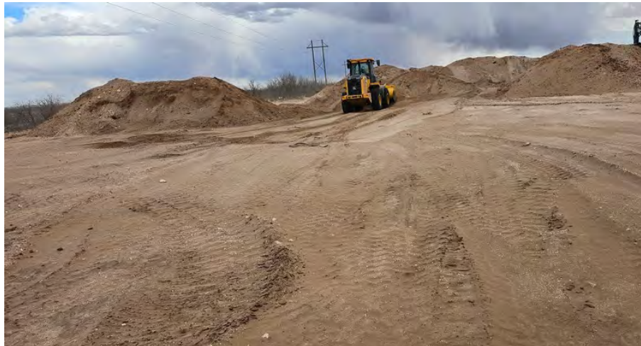
Figure 3: View of stockpiled caliche facing southwest from the northern extent of site. Date Taken: 2024-03-26 15:03:44. GPS: 32.3893943, -103.1902899
