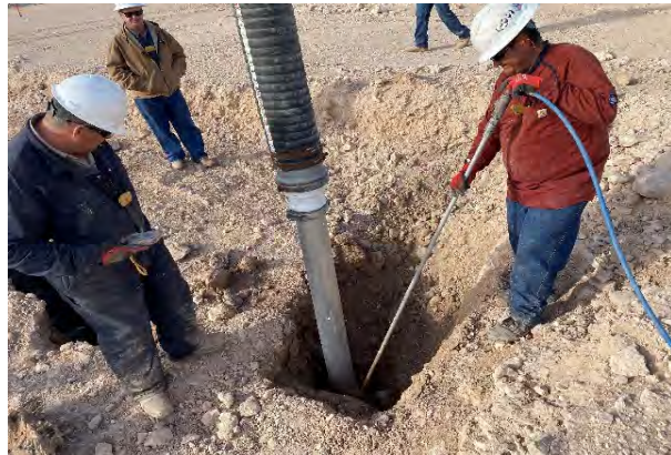
Photograph 5 Date: November 22, 2021 Description: View of field pothole 13, collected in open excavation and not submitted for laboratory analysis. Collecting samples at 3 feet and 4 feet was extremely difficult. Hydrovac hit refusal at 4 feet.
