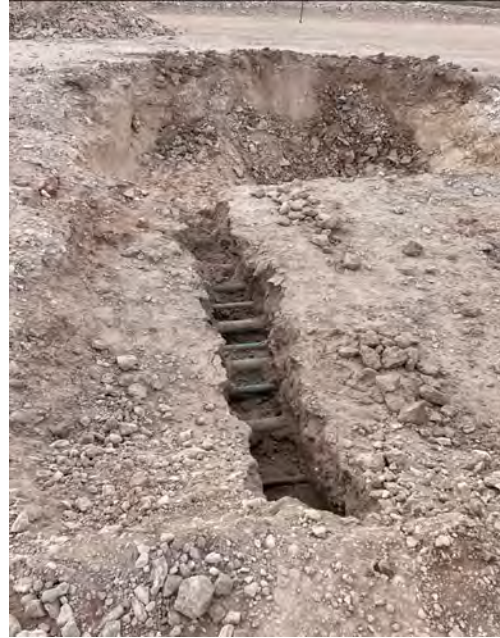
Photograph 2 Date: November 23, 2021 Description: View of spotting trench within the excavation. Several of the eleven lines are visible.
