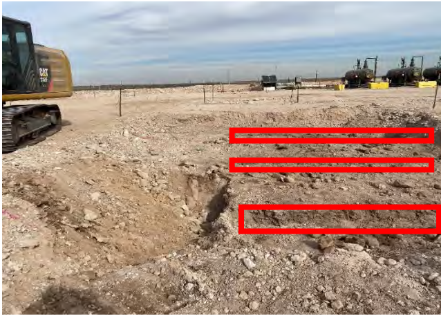
Photograph 1 Date: November 23, 2021 Description: View of excavation above the pipeline corridor facing north. The red outlines highlight trenches utilized to spot the six subsurface lines.
